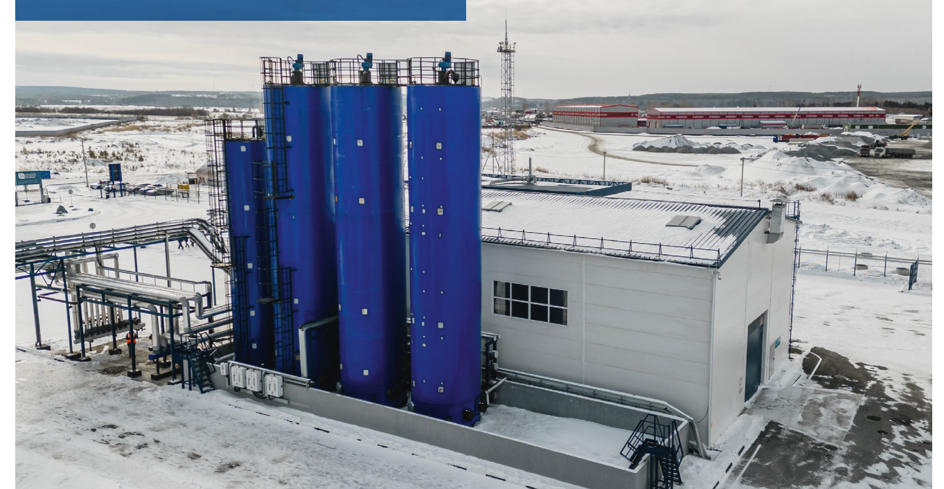
Mobile heating tanks ErichHahn MT
